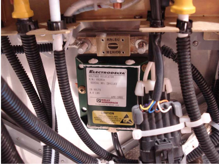
Figure 4 – Approximate location of VR-202A Voltage Regulator.
